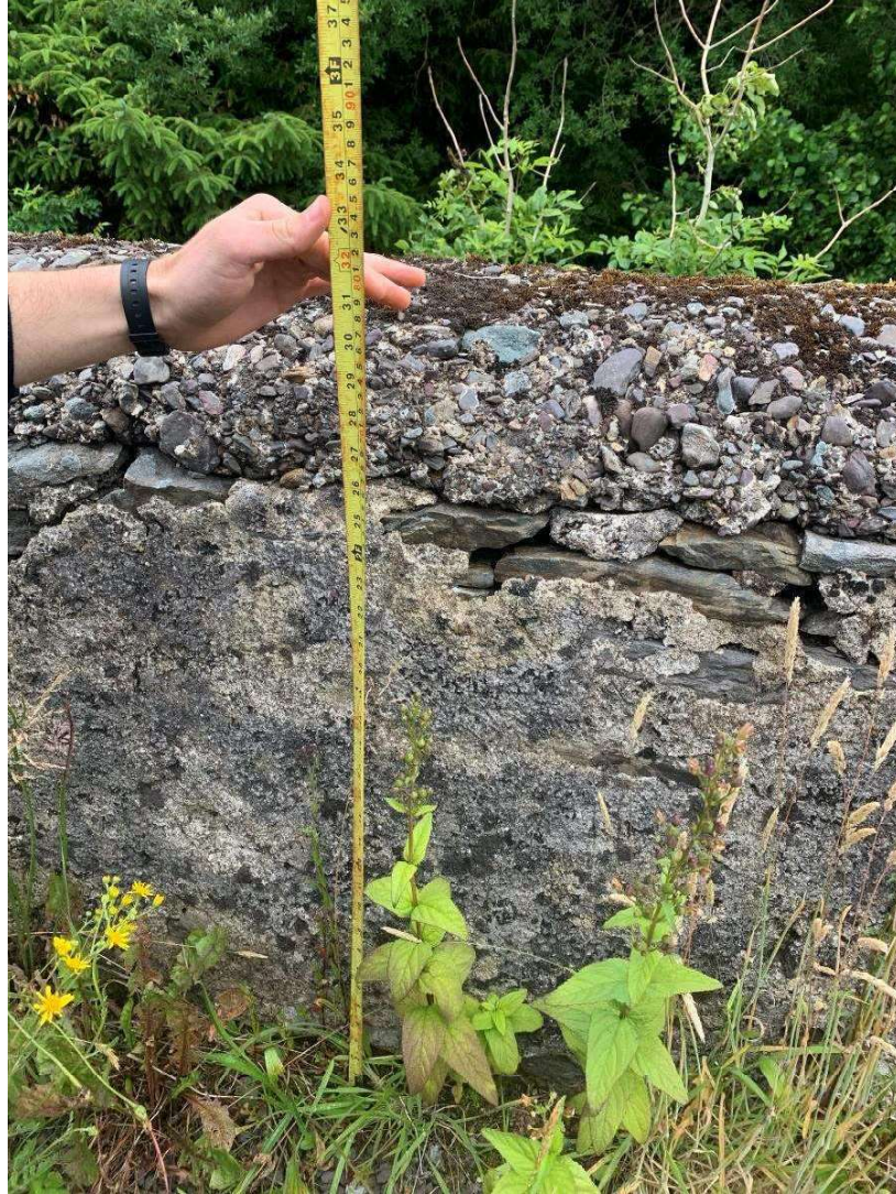
Parapet with concrete coping and repairs, open joints in exposed masonry
