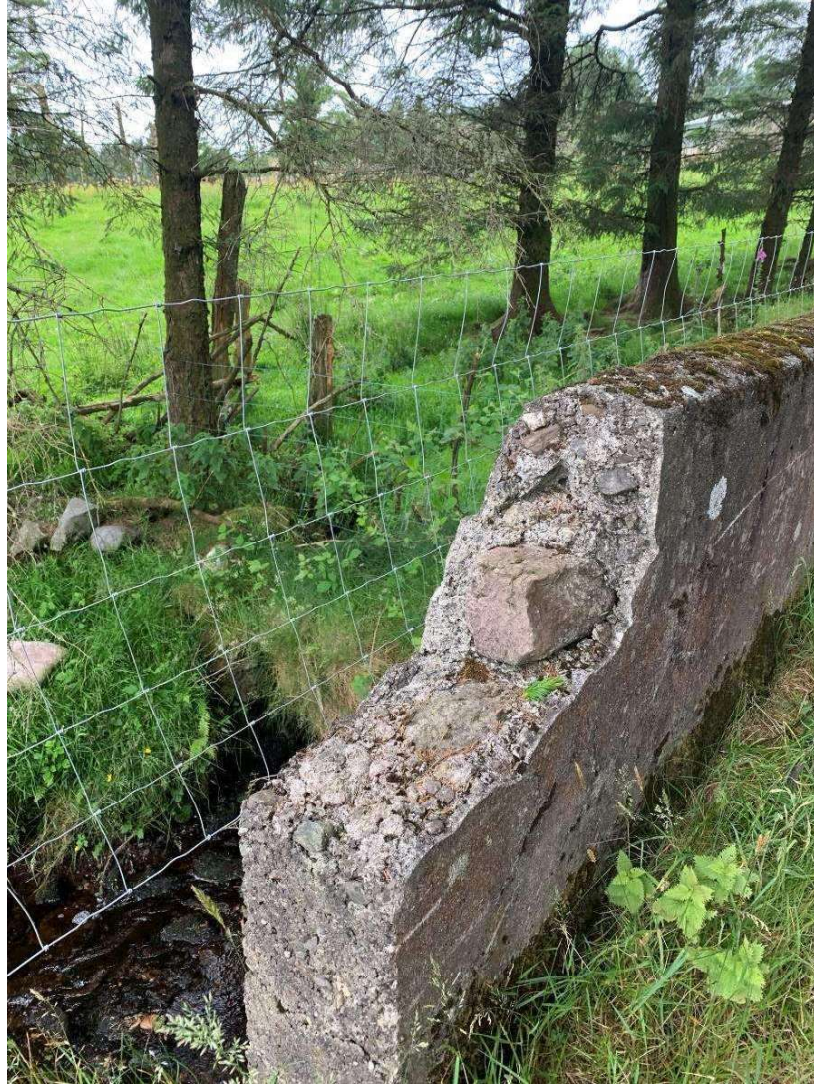
Knocked section of the downstream parapet
