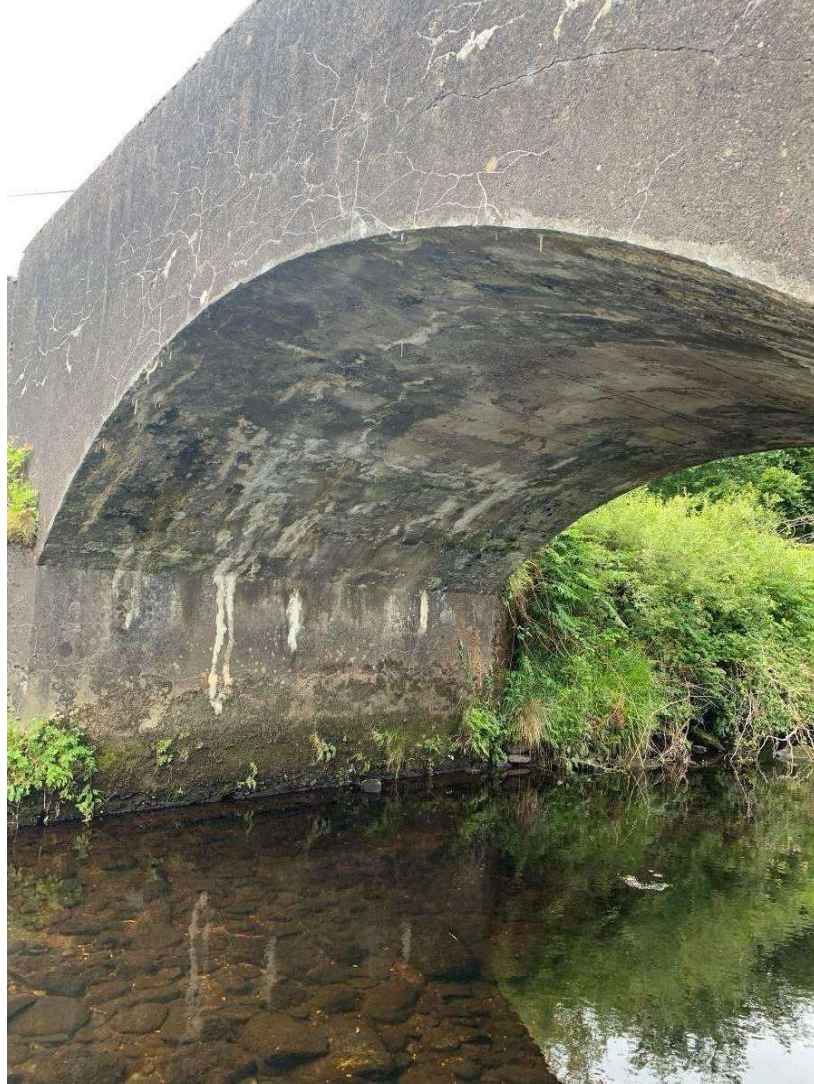
General view of bridge span showing typical condition of arch barrel and abutment
