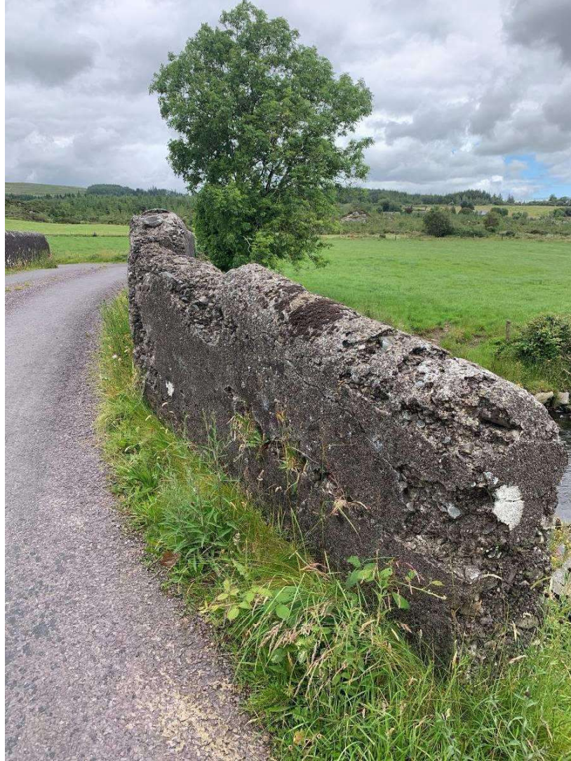
Close up of parapet showing concrete damage
