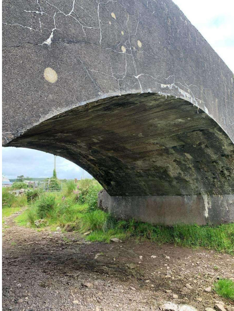
General view of bridge span showing typical condition of arch barrel and abutment
